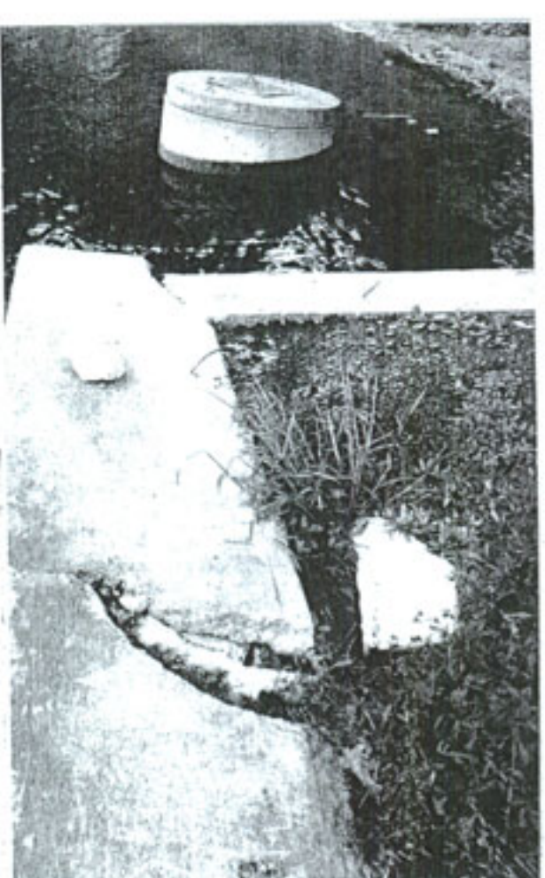
Photo F 'Shore well' now exposed and subject to ice damage
